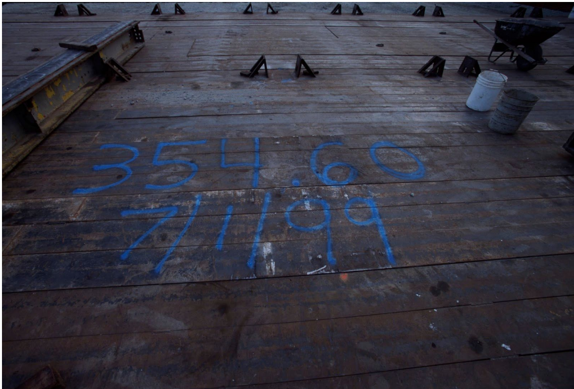
On July 1st, 1999 the Cape Hatteras Lighthouse was pushed 354.60'—the single day record for the move. (NPS photo)
